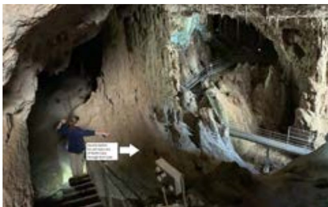
8. Location of new connection from Nettle Cave to Arch Cave, minimising impact by using the existing structure
