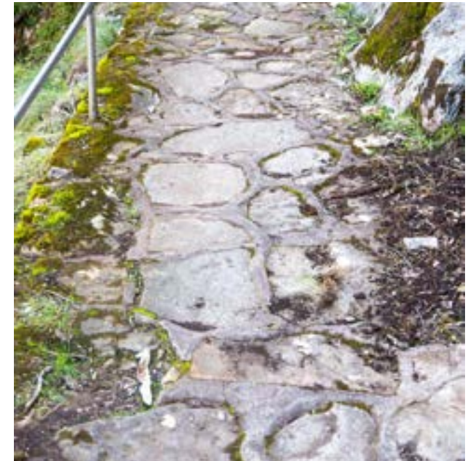
Section of the Six Foot Track to be upgraded to a concrete path.
