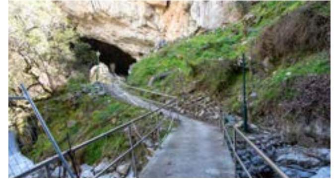
Damaged handrails from rockfall near Devils Coach House entrance
