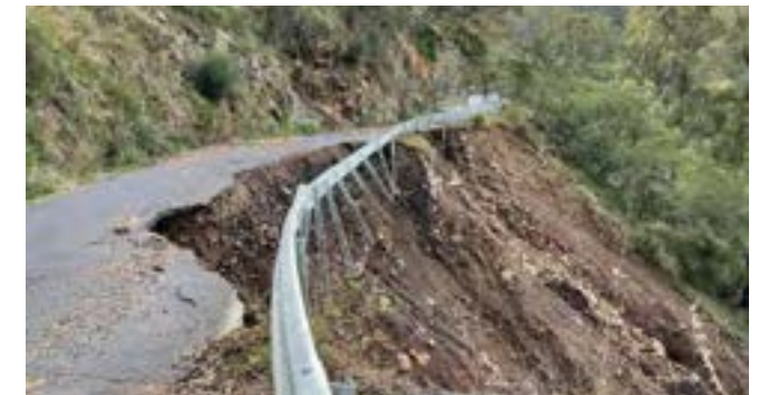
Landslip at Five Mile Photo: WSP
